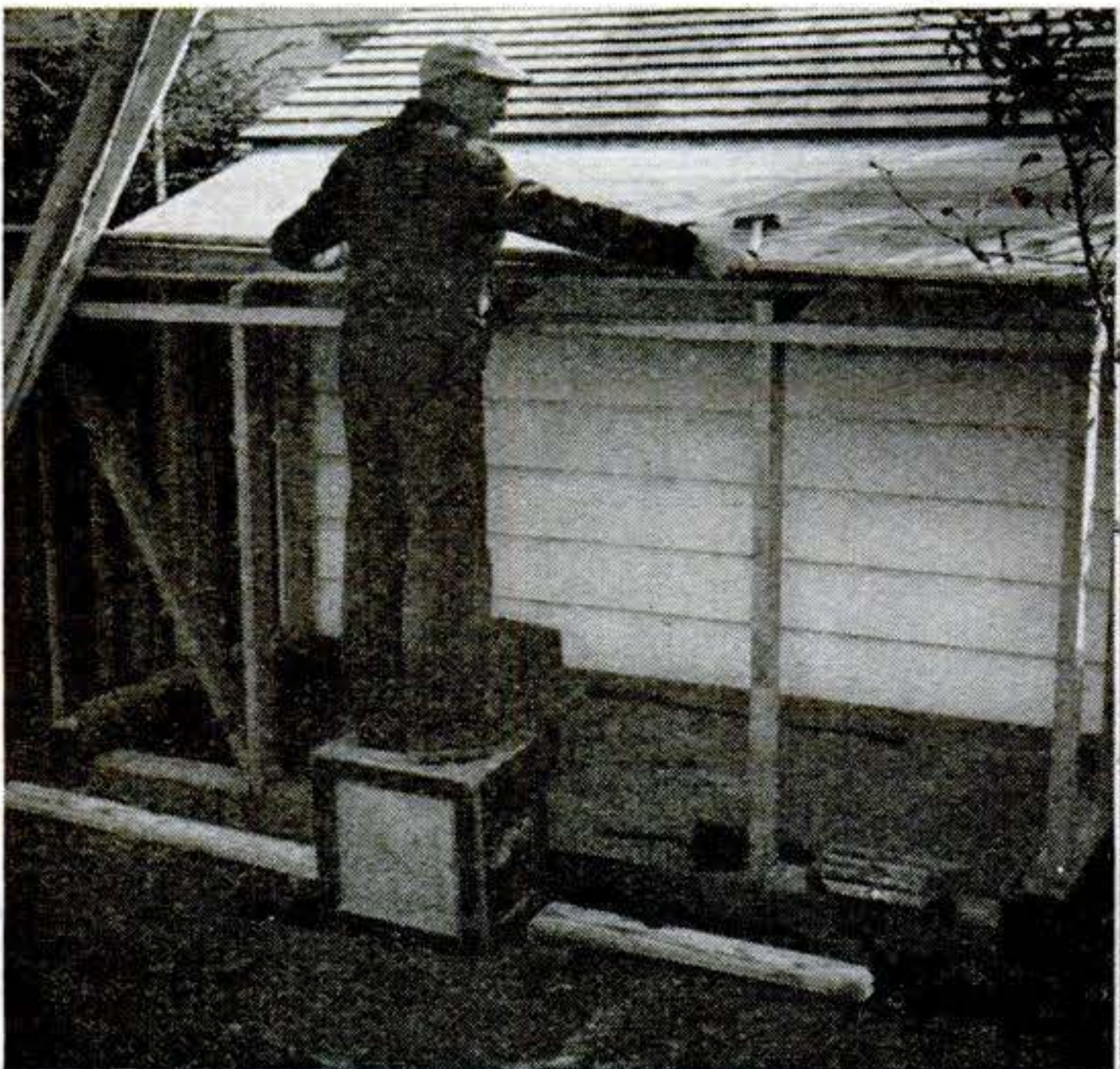
5 ROOF BOARDS laid over rafters are 1" by 6" tongue-and-groove. They overhang a little at sides and rear. Same stock is used to form sheathing on both sides.
